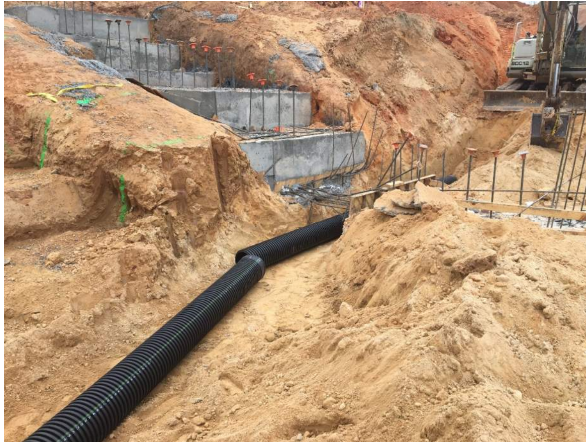
Storm Drain at Amphitheater Stairs
